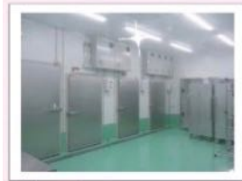
It is possible to utilize existing the refrigeration chamber.
